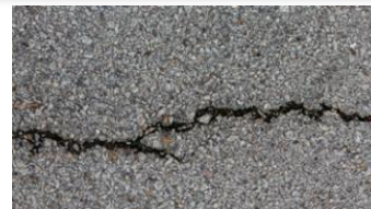
Pavement distress identification
